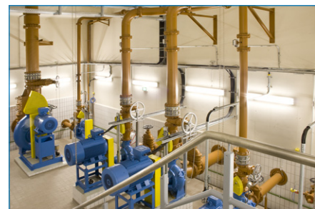
Blick in das Pumpwerk
